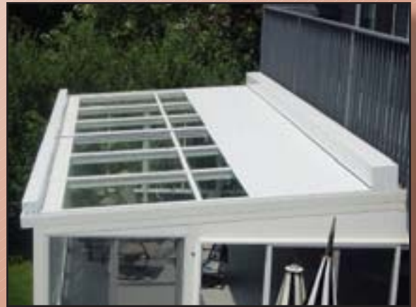
Push-Pull Shutter on Sunroom Roof
