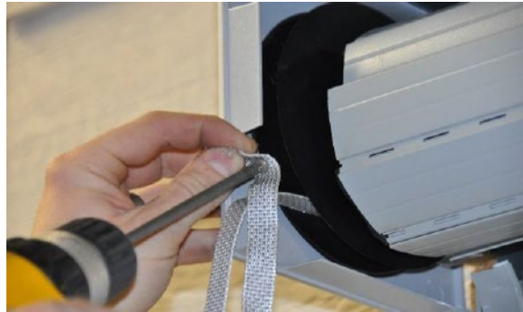
Screw strap to reel. Best to do with 2 screws. Roll shutter axle to wrap as much strap as possible onto the outside reel.
