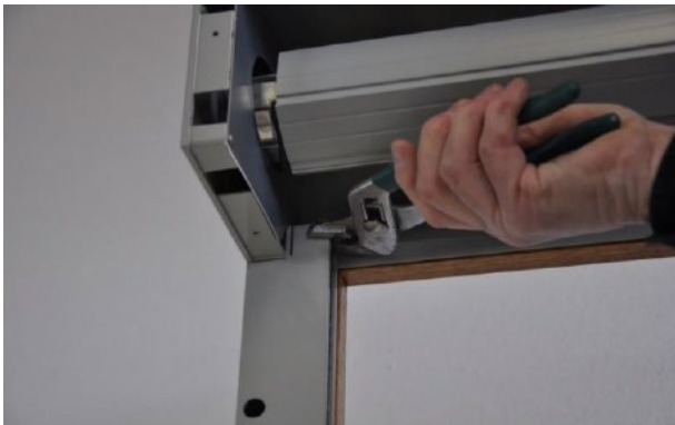
With channel lock pliers bend front ear of tracks out 30 degrees to form guide.
